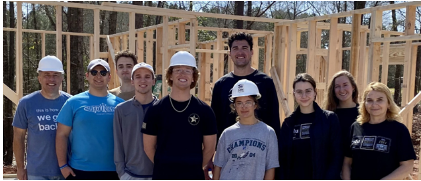
Dr Mistrean (far right) and Dr Saunders (far left) along with undergraduate business students framing walls during a Habitat for Humanity workday in March 2024.
